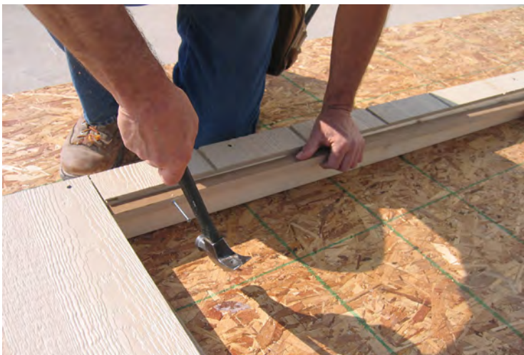
17. Next install door stops as shown. Keep flush with the top of 2x4 (not the Smartside) and secure with 2" nails.
