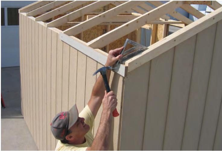
61. Next, install 2 3/4" trim as shown, keep flush with the outside of the rake and fasten with 2" nails.
