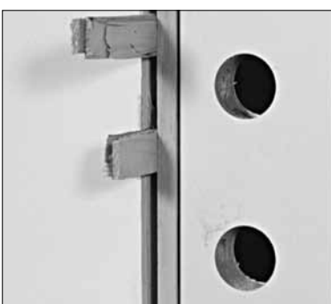
Figure 14: Shims are placed above and below the dead bolt hole (points G in figure 12).
