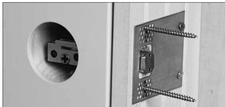
Figure 27: Screws should connect the dead bolt plate to the stud.
