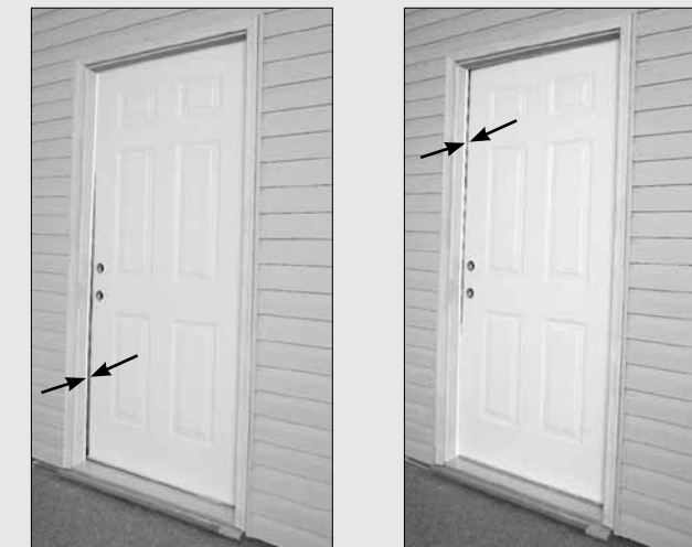
Figures 9 and 10: The weatherstripping on these doors is not evenly compressed.
