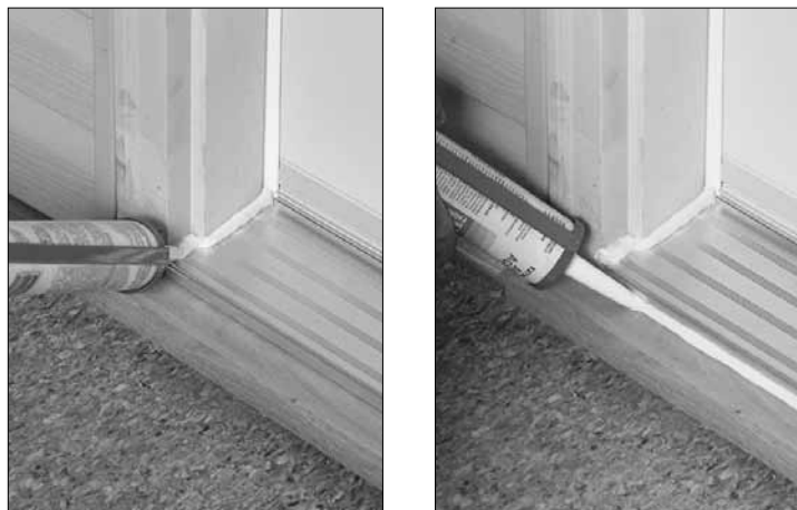
Figures 29 and 30: Caulk the sill crown and the front of the sill.
