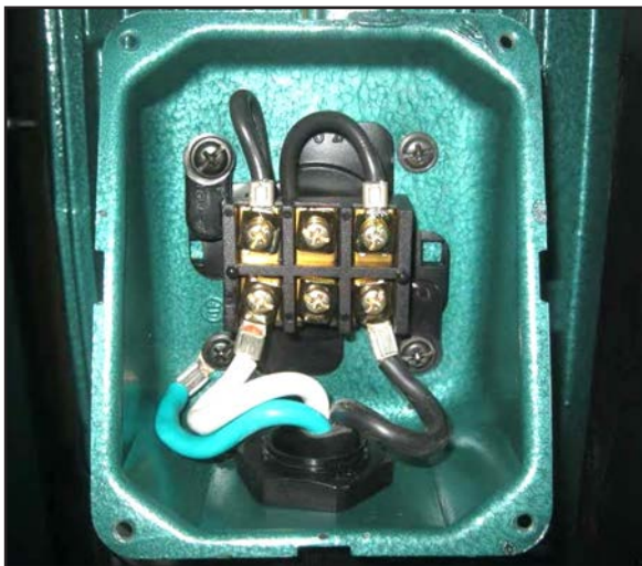
Figure 50. G0671 motor junction box.
