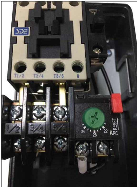
Figure 49. G0671 MA-15 contactor.
