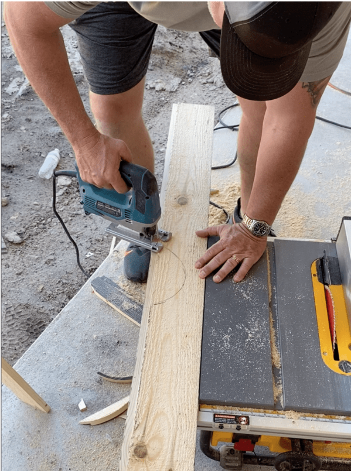
Jason using a jig saw to cut a hole for a can light.
