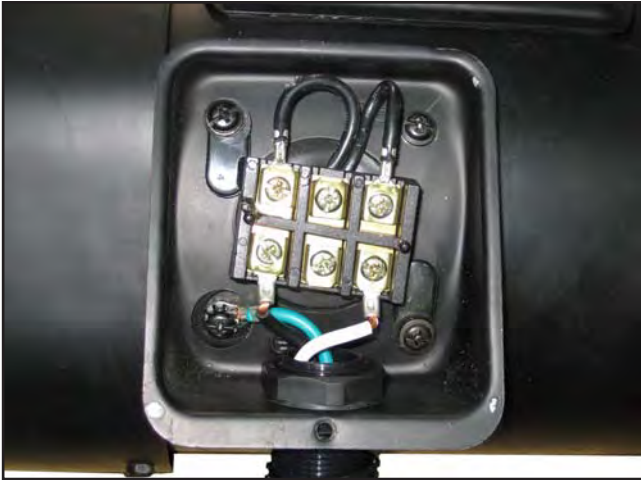
Figure 147. G0651 motor junction box.
