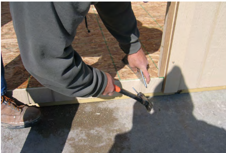
74. Install kick plate. Keep flush with top of floor and fasten with 2" nails.
