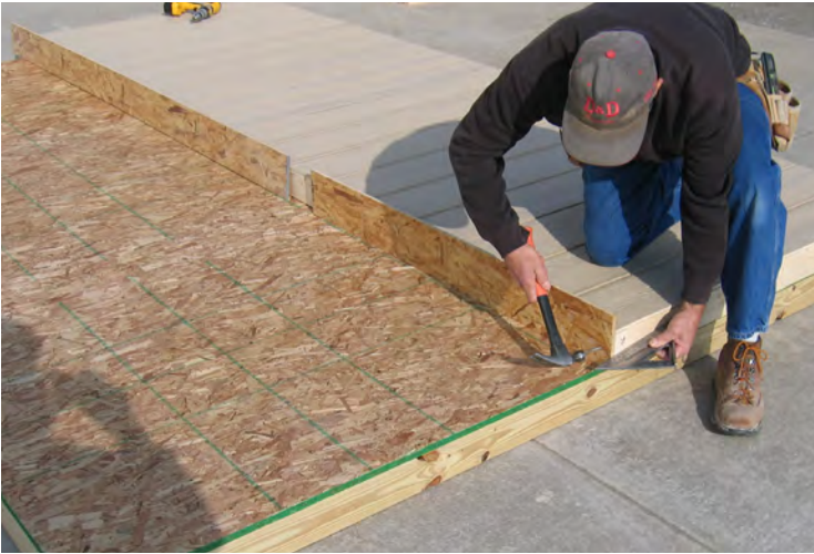
13. Make sure the OSB top plate is flush on the bottom side (inside of wall), and the side.
