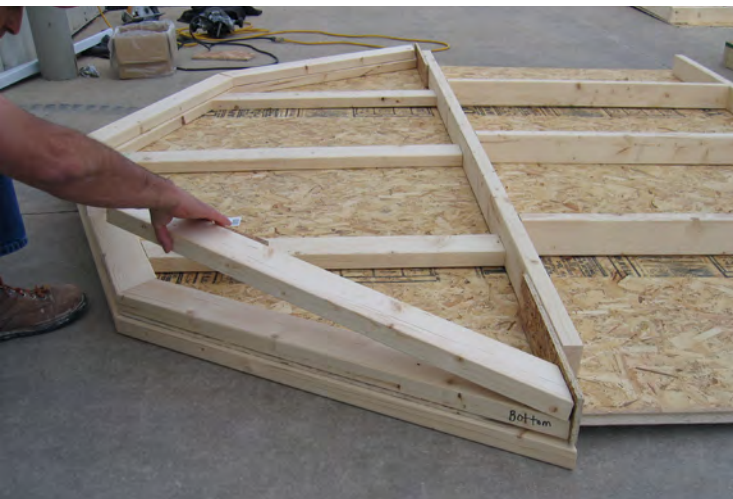
58. Next locate all truss parts, and using the previously assembled gable truss, as a template, layout the trusses.
