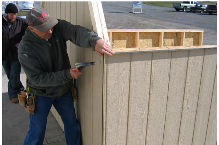
69. Make sure the walls fit nice and tight and fasten with 2" nails every 8".
