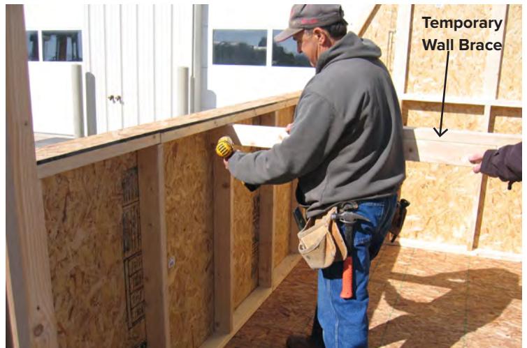
77. The temporary wall brace will be removed when building assembly is completed.
