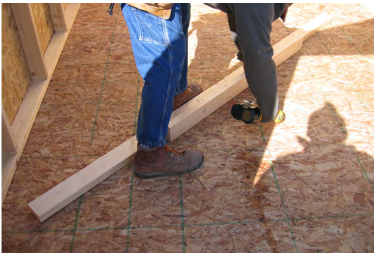
76. Space wall braces according to width of the building and attach with 2 1/2" screws.
