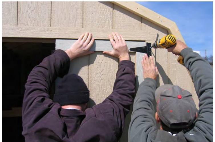
93. For door installation, you will be using three hinges, per side. Use one 2 1/2" blackheaded screw, per hinge. Fill the remaining screw holes with 1 1/4" screws. This is done for both sides.
