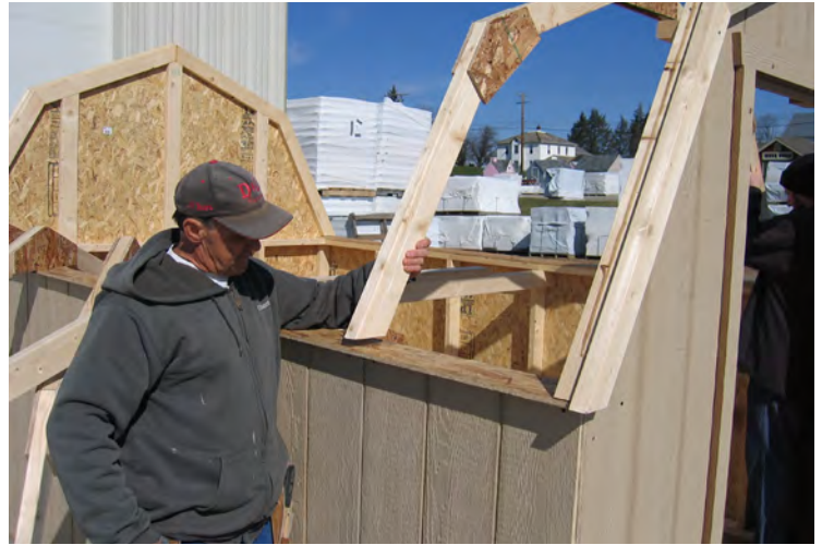
79. Install trusses, as shown, making sure they are 24" on center before fastening.
