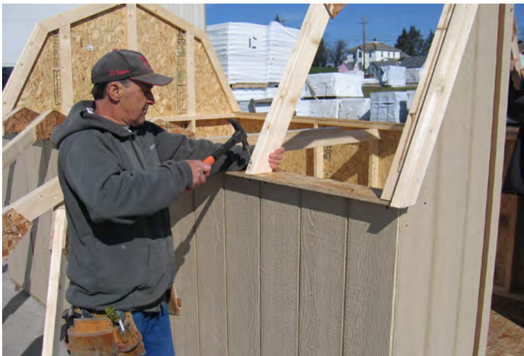
80. Secure with 3" nails where marked. Put a nail on each side and on the front.
