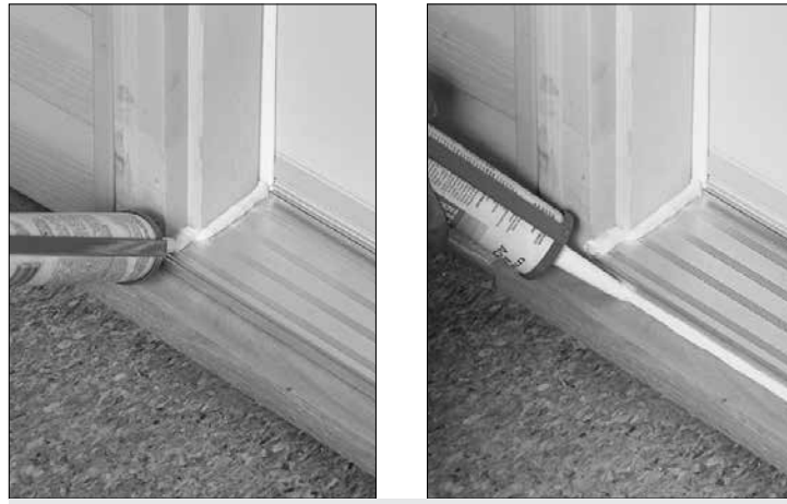
FIGURES 24 and 25: Caulk the sill crown and the front of the sill.
