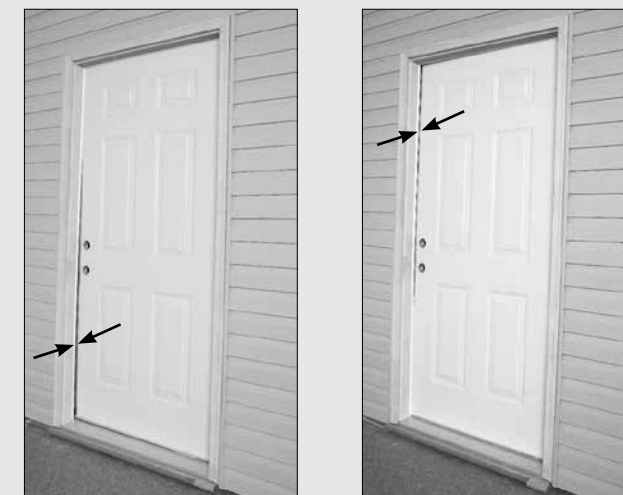
Figures 8 and 9: The weather-stripping on these doors is not evenly compressed.
