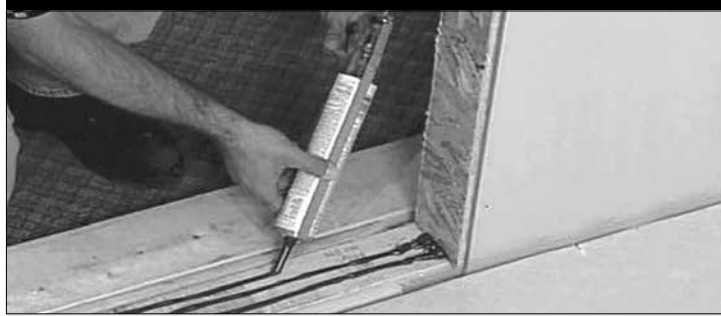
FIGURE 2: Caulk is applied in three parallel lines running the width of the sill.
