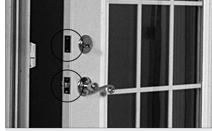
FIGURE 29: The latch and dead bolt are installed per the hardware manufacturer installation detail.
